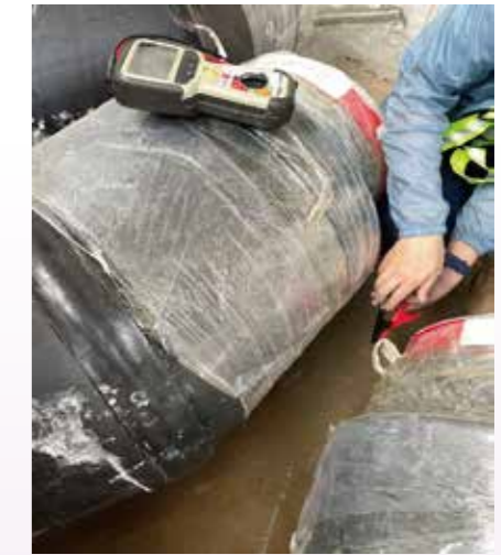
Figure 8. U/G Water Leakage Cabling Joints
